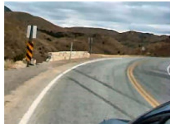
A car has skidded while rounding a corner, tangent to the double yellow lines curve.
